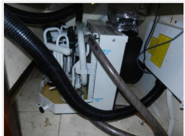
New air conditioning unit
