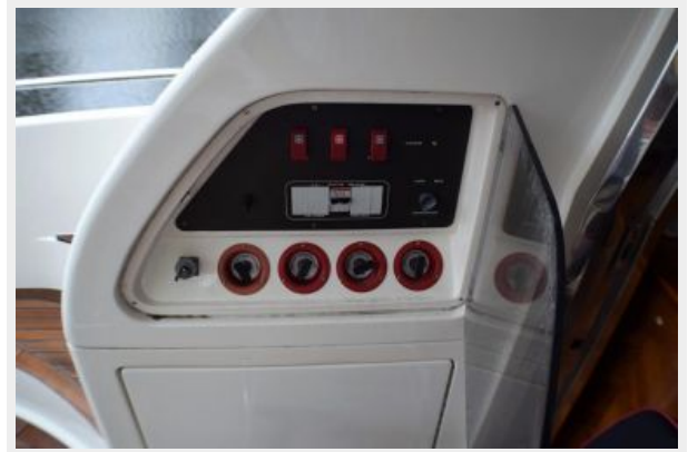
Battery Control Panel
