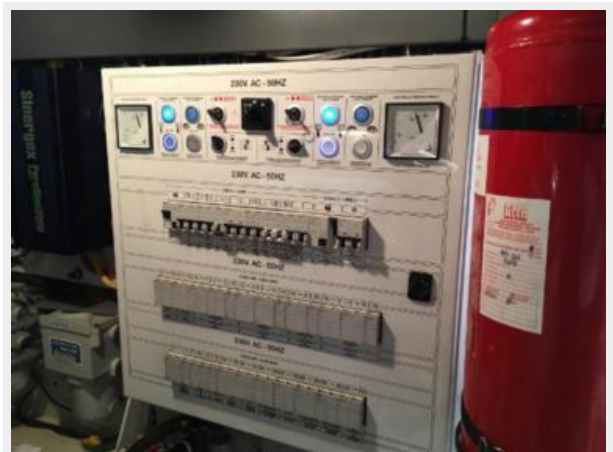
Main Distribution Panel
