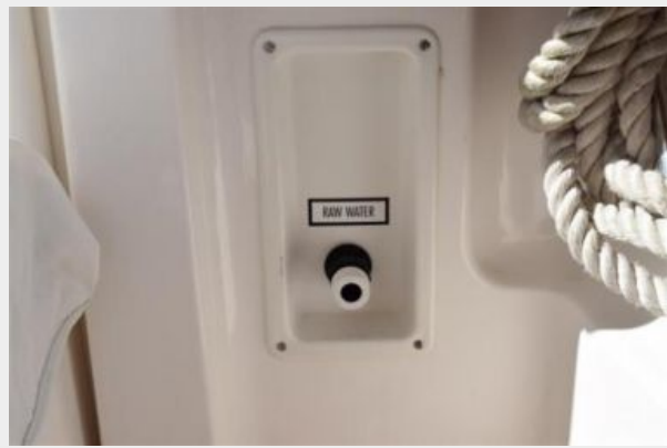
Raw Water Connection
