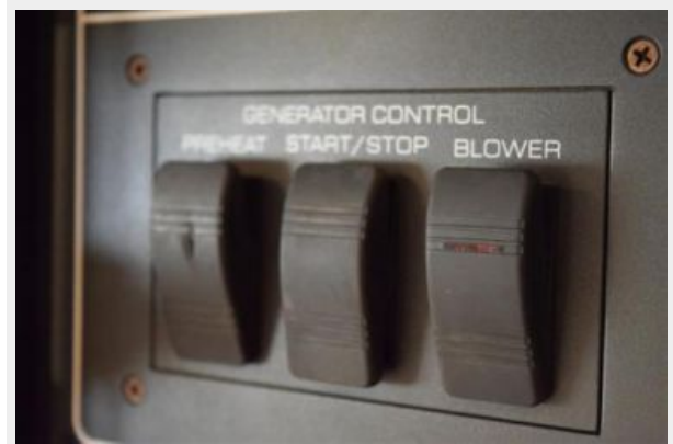
Generator Control Panel
