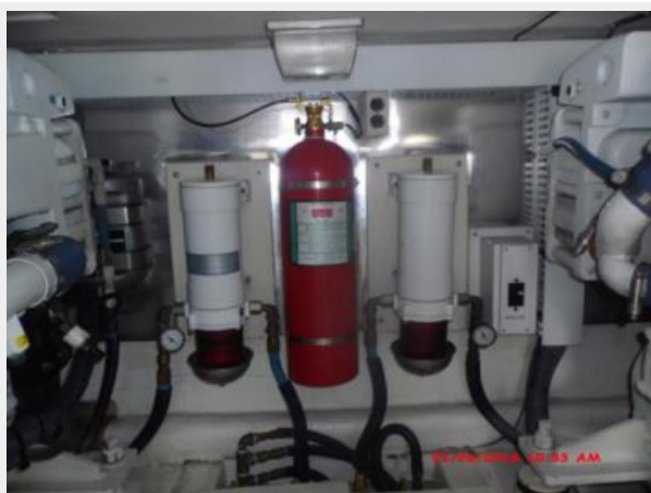
Engine & Mechanical Equipment 5 - Fire Control System
