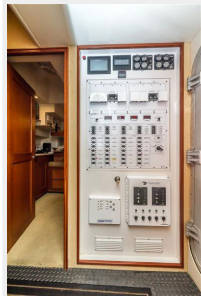
Electrical Distribution Panel
