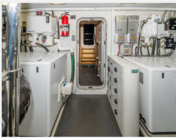
Engine Room Generators
