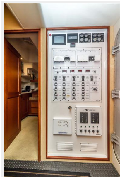
Electrical Distribution Panel
