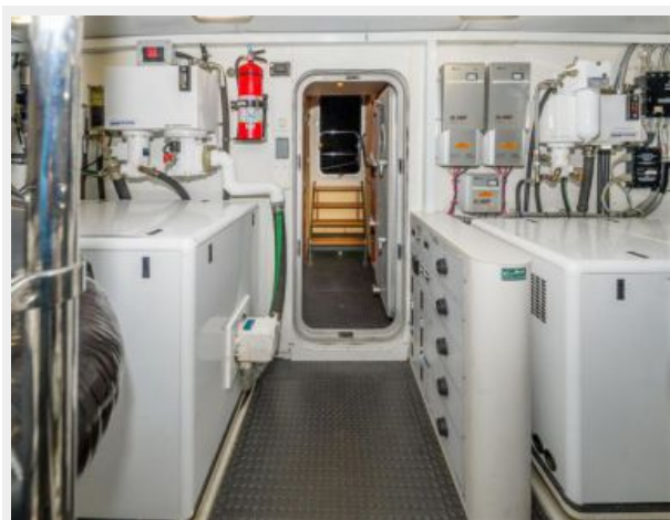
Engine Room Generators
