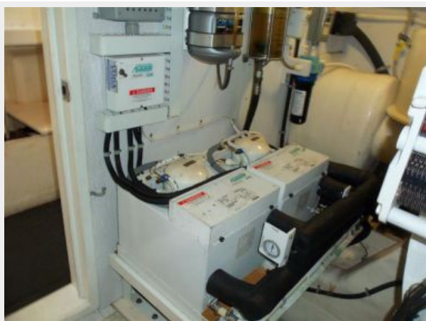
Chilled Water AC
