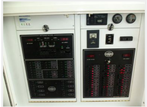
Helm Electrical Panel
