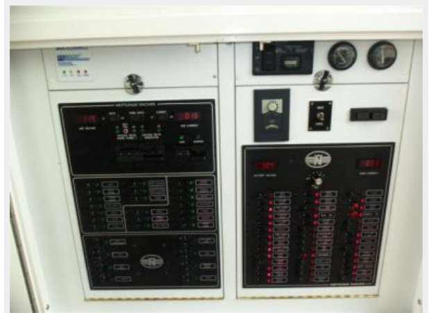
Helm Electrical Panel
