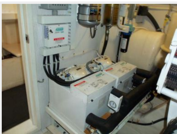
Chilled Water AC
