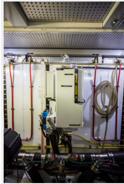
Centerline Fuel Tanks with Site Tubes, Hydraulics
