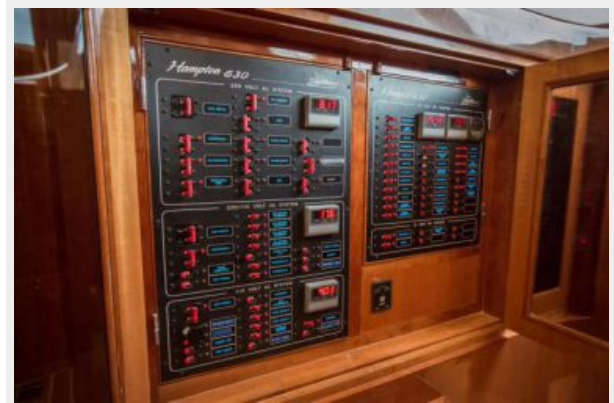
Hampton 63 Electrical Panel, Companionway
