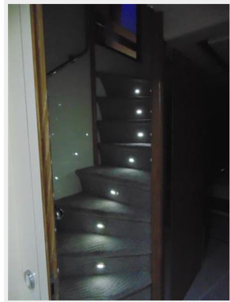
New LED Lighting
