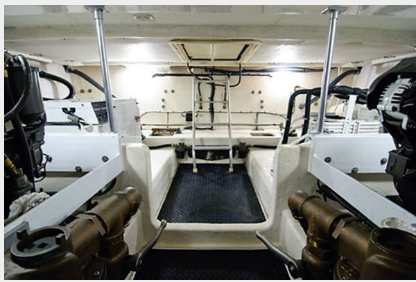
Engine Room Looking aft
