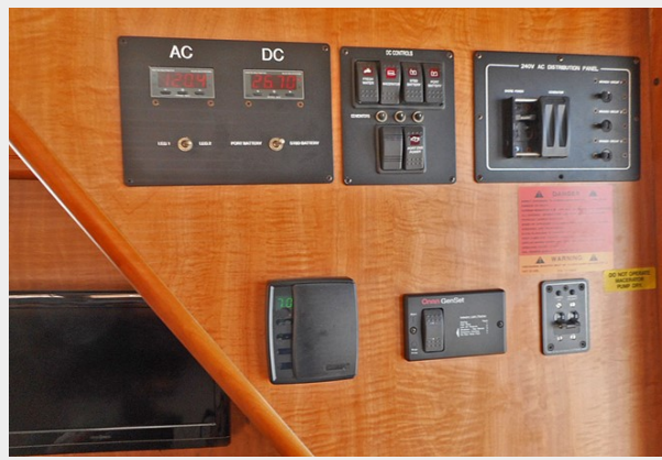
Electric Panel-Easily accessible at salon entry
