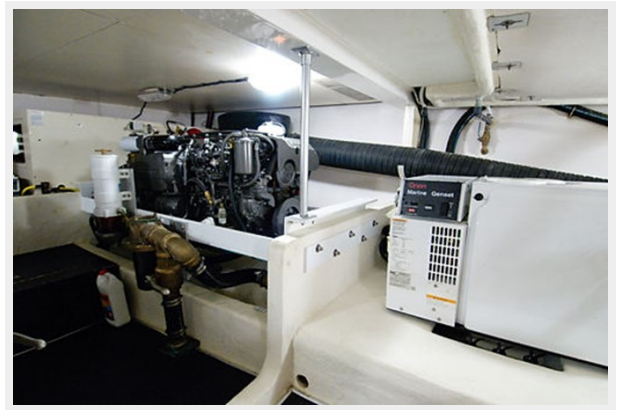
Engine Room-9 KW Onan Generator with Sound Shield and Starboard Engine
