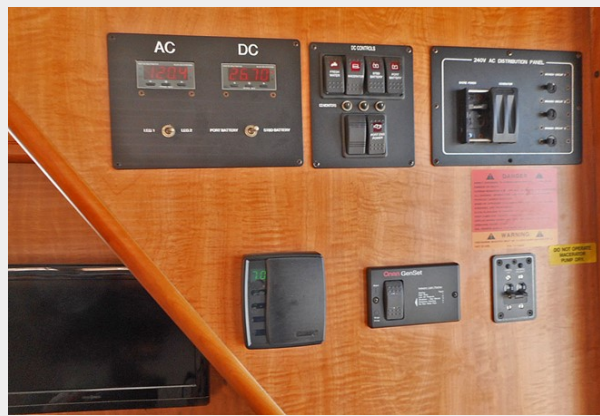
Electric Panel-Easily accessible at salon entry
