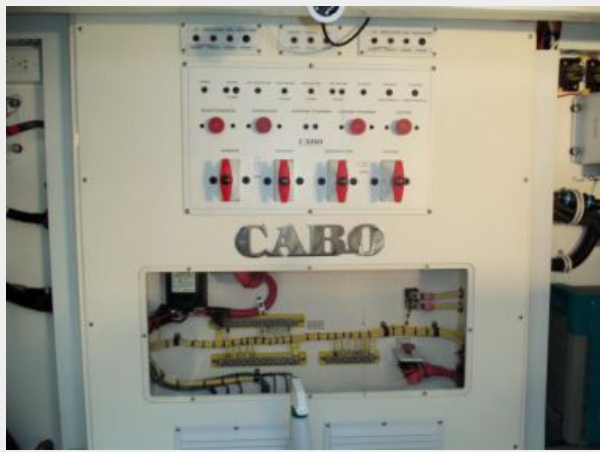
Engine Room Panel
