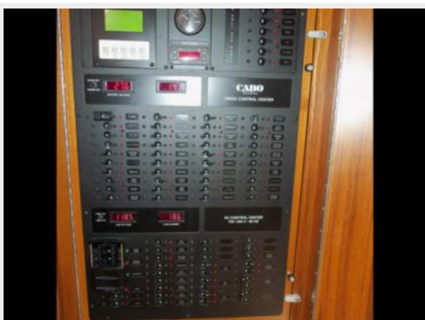
Main Electrical Panel
