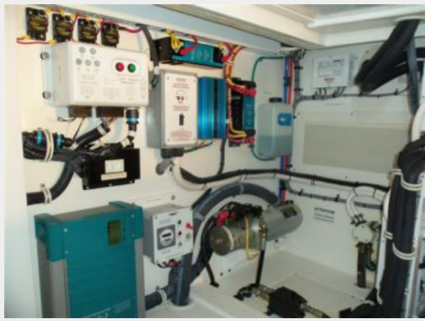
Engine Room Forward
