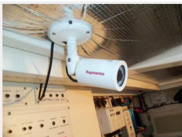
Engine Room Camera
