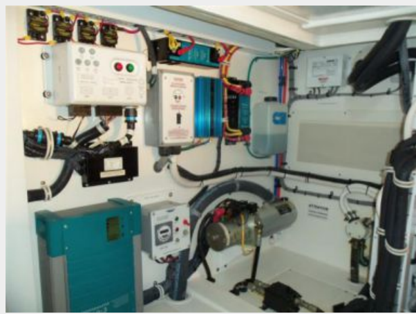
Engine Room Forward
