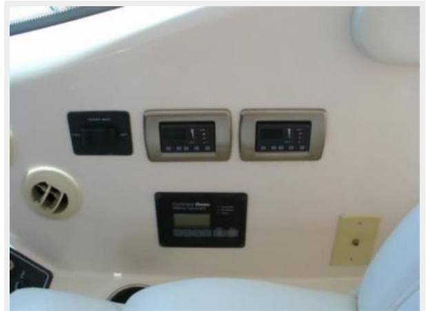
Cockpit Air Conditioning Controls
