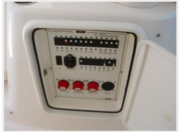
Cockpit Circuit Breaker/Battery Panel
