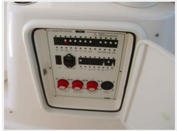
Cockpit Circuit Breaker/Battery Panel
