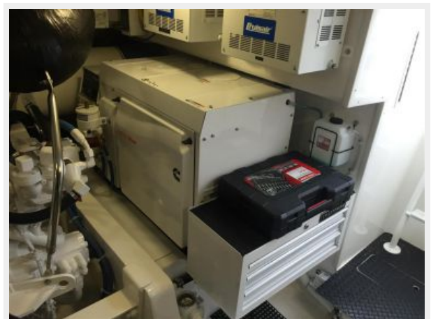
Electrical Equipment - Onan Generator #2
