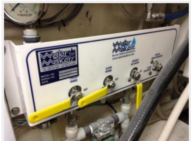
Water make Control 2
