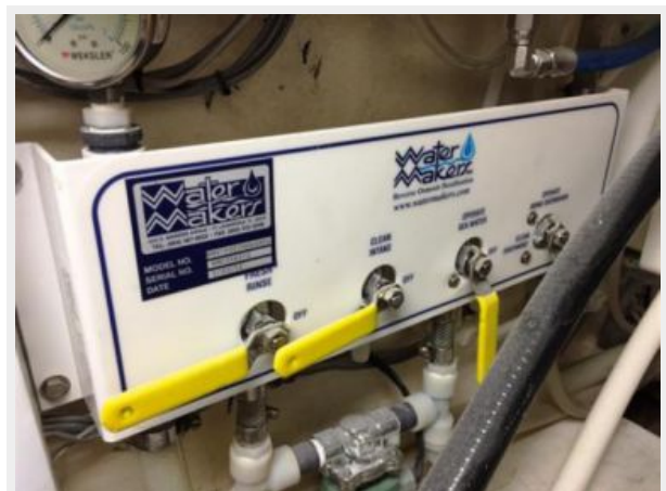
Water make Control 2
