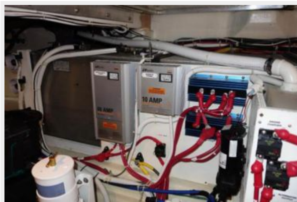
Battery Chargers and tanks
