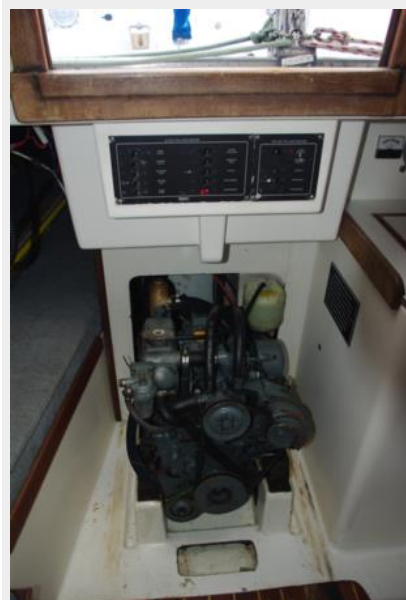
Engine box (exposed)
