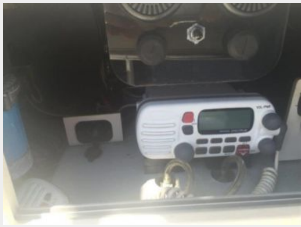
VHF in Tower
