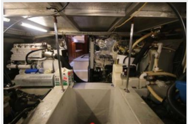
engine room looking forward
