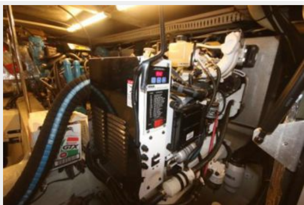
Kohler genset, 10KW
