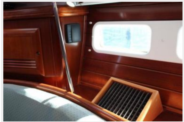
Salon Air Conditioning Supply Vent
