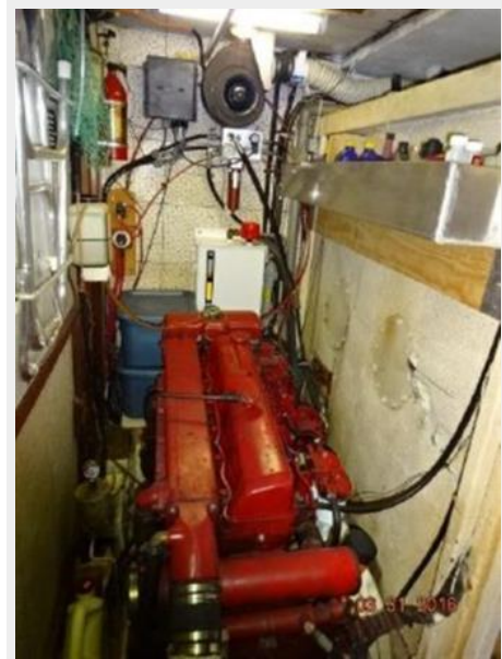
50' Marine Trader starboard engine room
