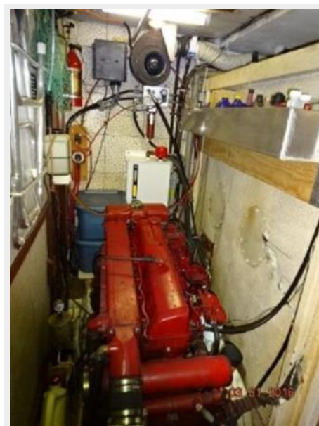
50' Marine Trader starboard engine room
