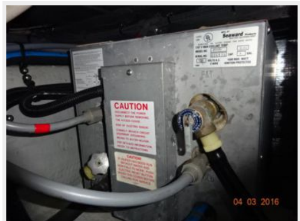
37' Mainship water heater
