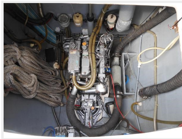
starboard engine room
