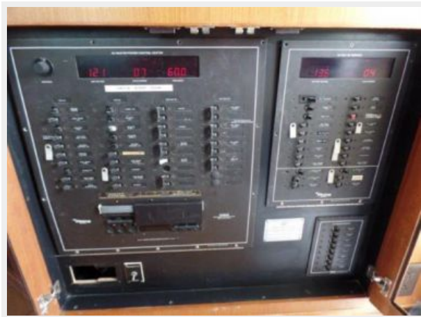
Main Breaker Panel
