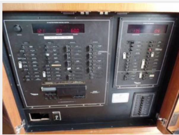
Main Breaker Panel
