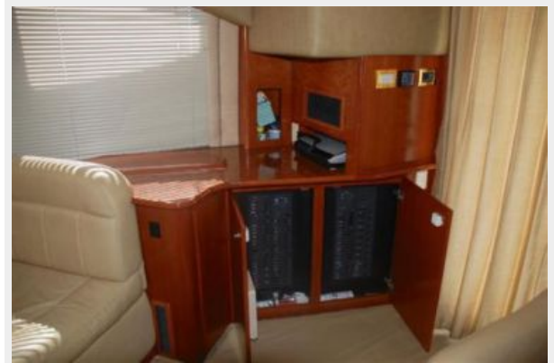
Power Breaker Station
