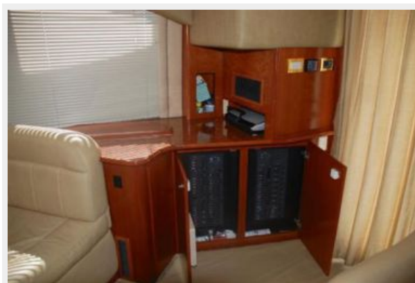
Power Breaker Station
