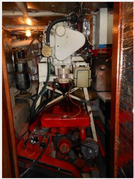
Generator above main engine
