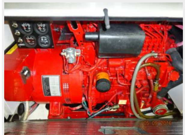
49' DeFever 12.5 kW generator
