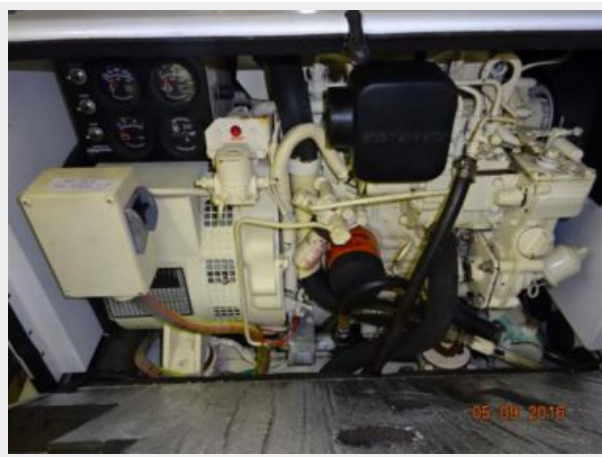
49' DeFever 5 kW generator
