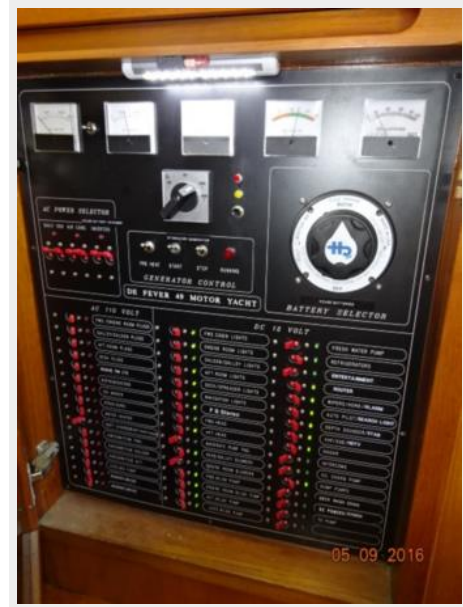
49' DeFever electrical panel
