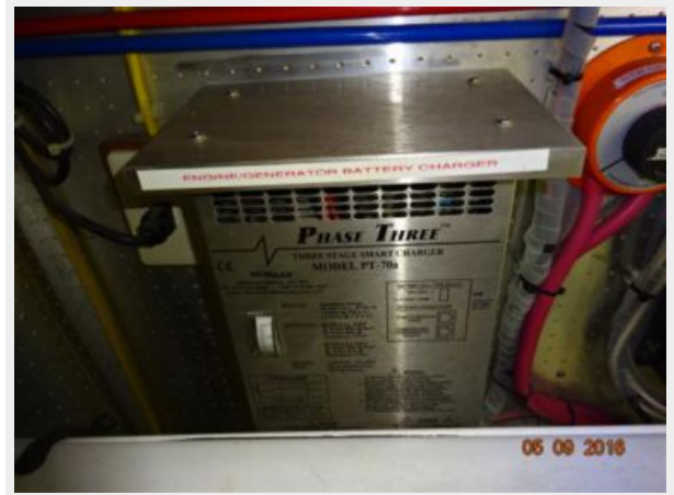
49' DeFever battery charger
