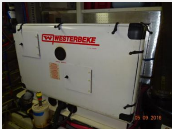
49' DeFever 12.5 kW generator soundbox
