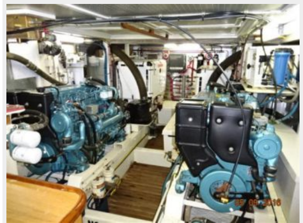
49' DeFever engine room aft
