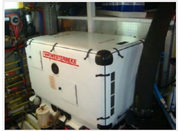
49' DeFever 5 kW generator soundbox
