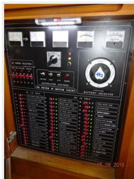
49' DeFever electrical panel
