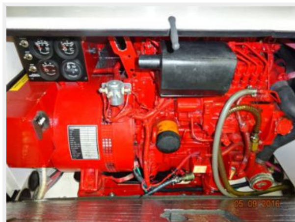
49' DeFever 12.5 kW generator
