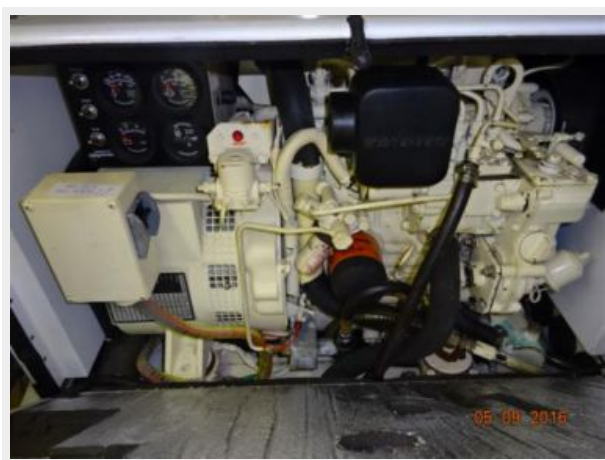
49' DeFever 5 kW generator
