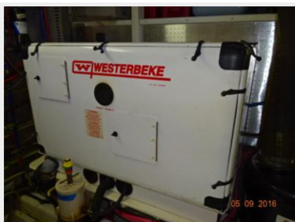
49' DeFever 12.5 kW generator soundbox
