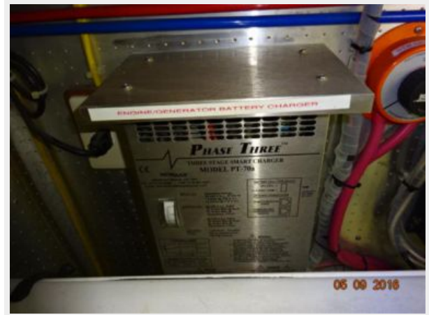
49' DeFever battery charger
