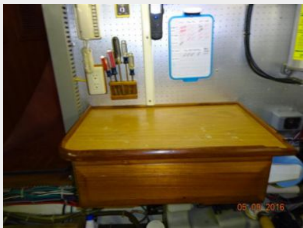
49' DeFever engine room work bench
