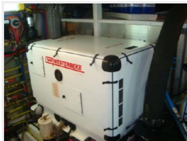
49' DeFever 5 kW generator soundbox
