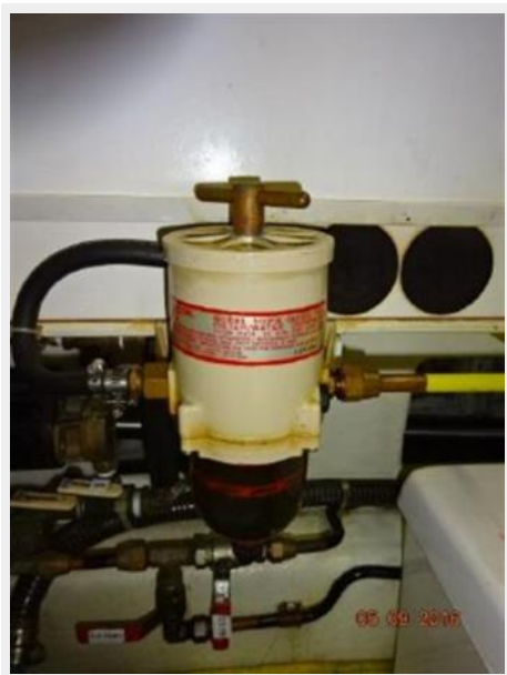
49' DeFever 12.5 kW generator Racor fuel filter
