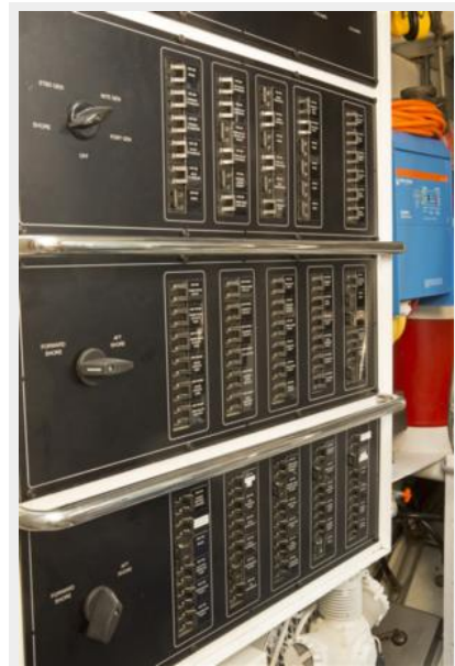
Main Electrical Panel in Engine Room
