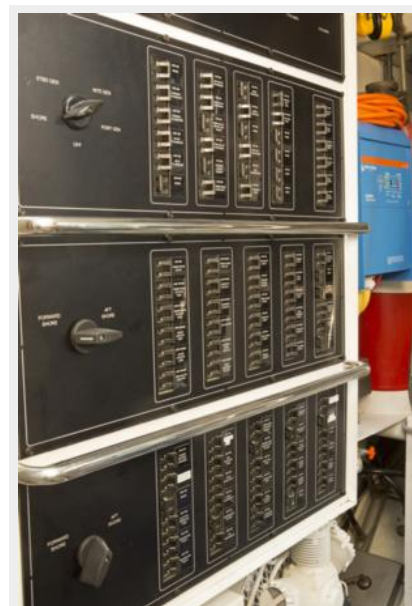
Main Electrical Panel in Engine Room
