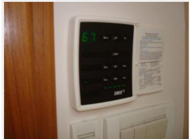
Digital AC controls
