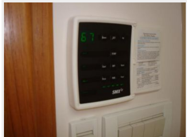
Digital AC controls
