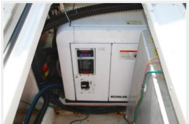
Kohler Generator Lazarette
