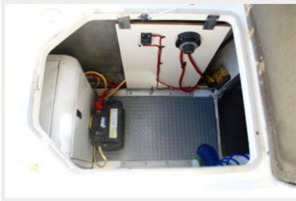
Engine Room Access
