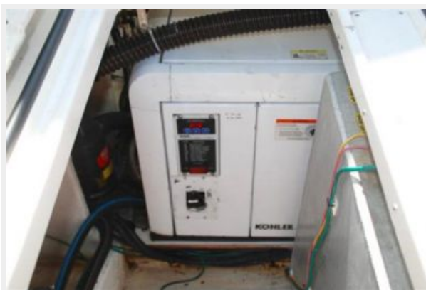
Kohler Generator Lazarette
