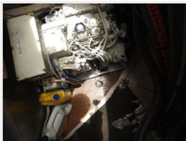
Northern Lights Generator with 9000 hours
