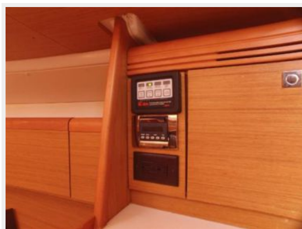
Galley A/C Control and Propane Control
