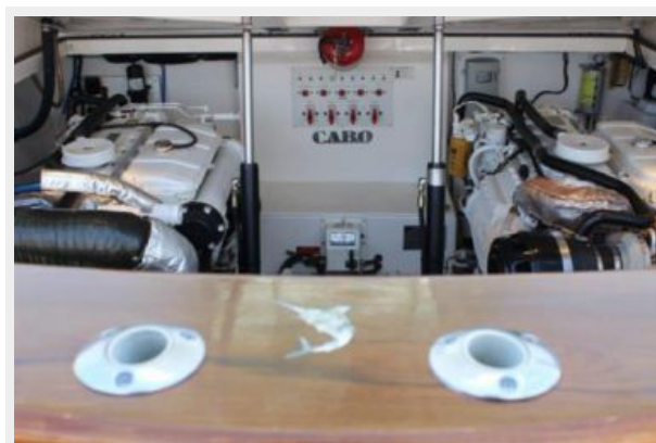
Engine & Mechanical Equipment 1 - Engine Room
