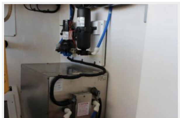
Engine & Mechanical Equipment 7 - Engine Room
