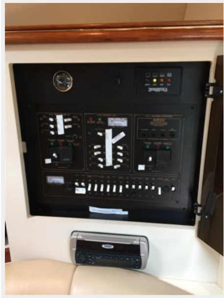
Main Distribution Panel
