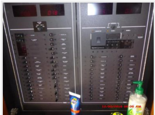
Electrical System / Equipment - Electrical Panel
