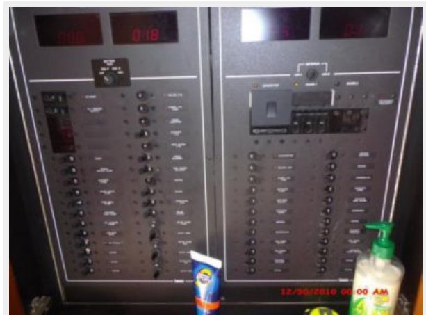
Electrical System / Equipment - Electrical Panel
