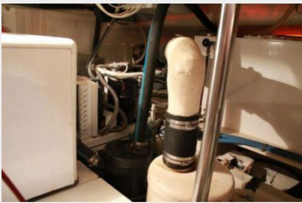
Remote AC & Port Fuel Tank
