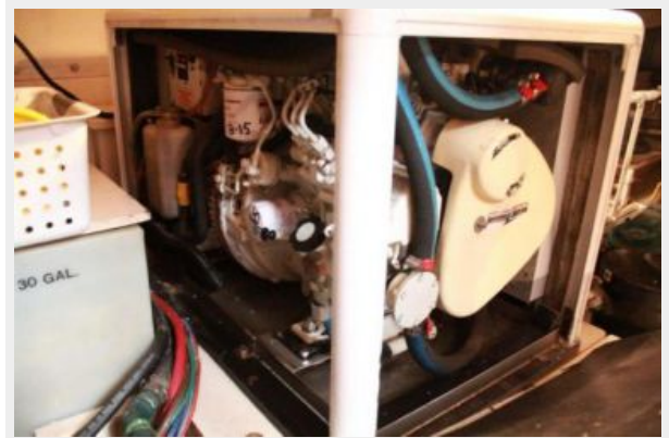
Northern Lights Generator
